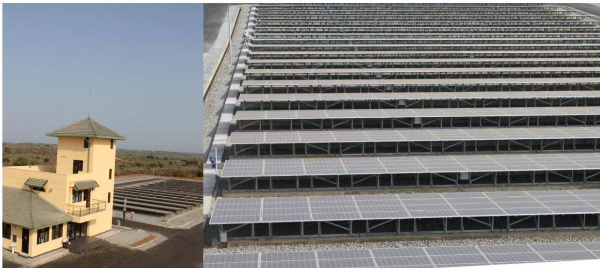
Figure 6: Solar plant Hambantota
