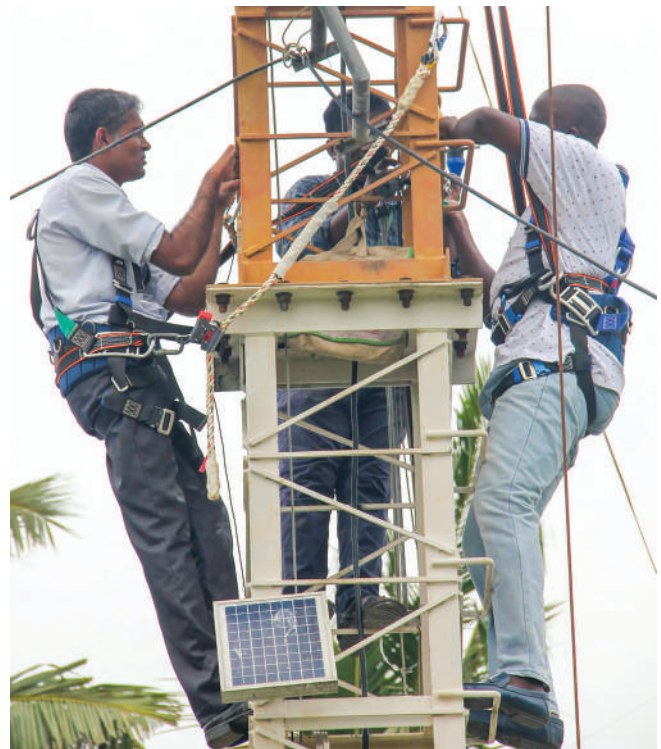
Wind Resource Assessment and Wind Farm Planning, National Institute of Wind Energy, India
