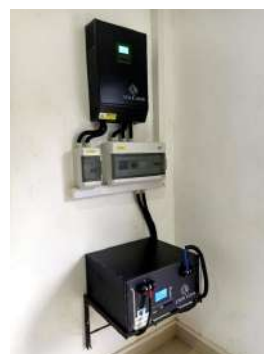
PV / ESS at Indurana site
