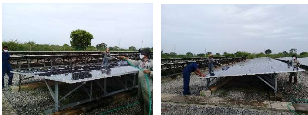
Cleaning of Solar Panels
